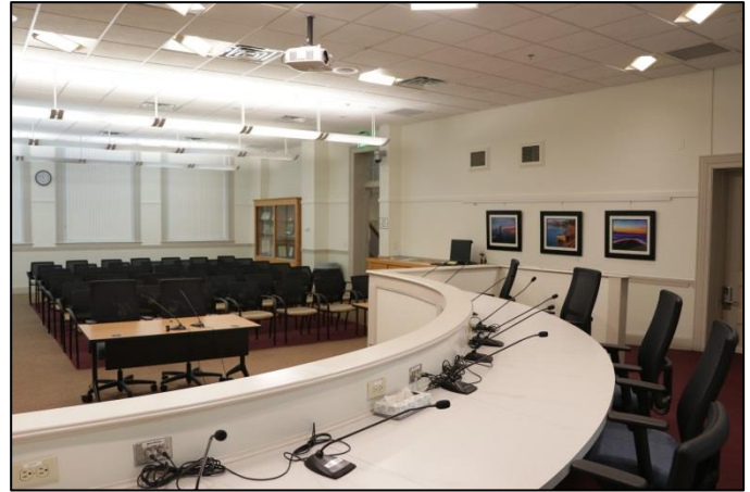
Electrical Components - Town Council Seating
