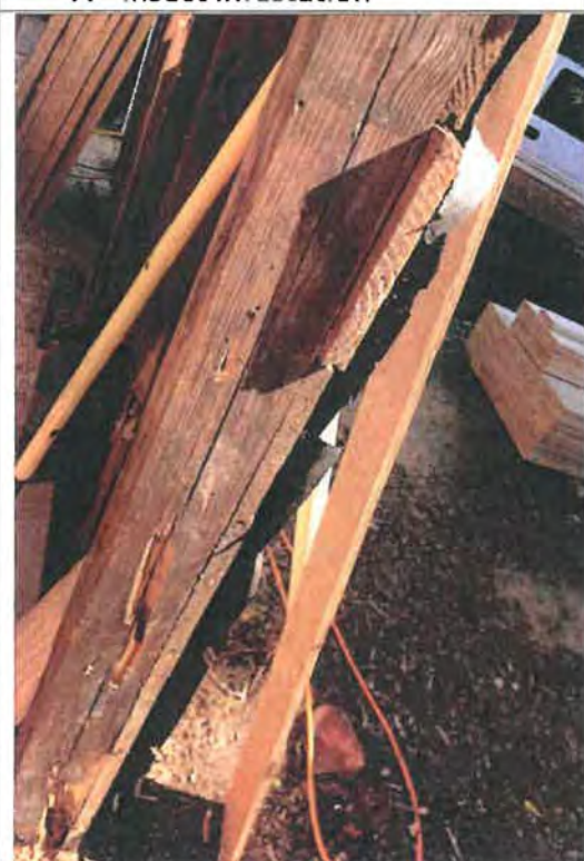
9. Carpenter ant infestation.
