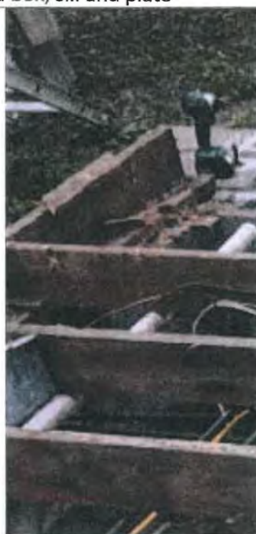
10. Rotted sills and box
