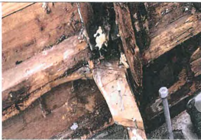
8. Rotted box, sill and plate
